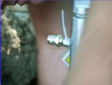
Open bleed off valve
